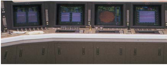
Picture 6 Overall view of operator console (upper: CRT, lower: FD)
