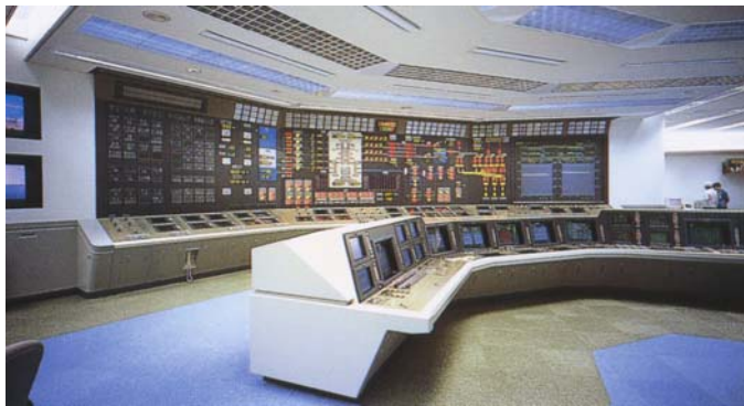
Picture-3(A): 3rd Generation Control Panel
